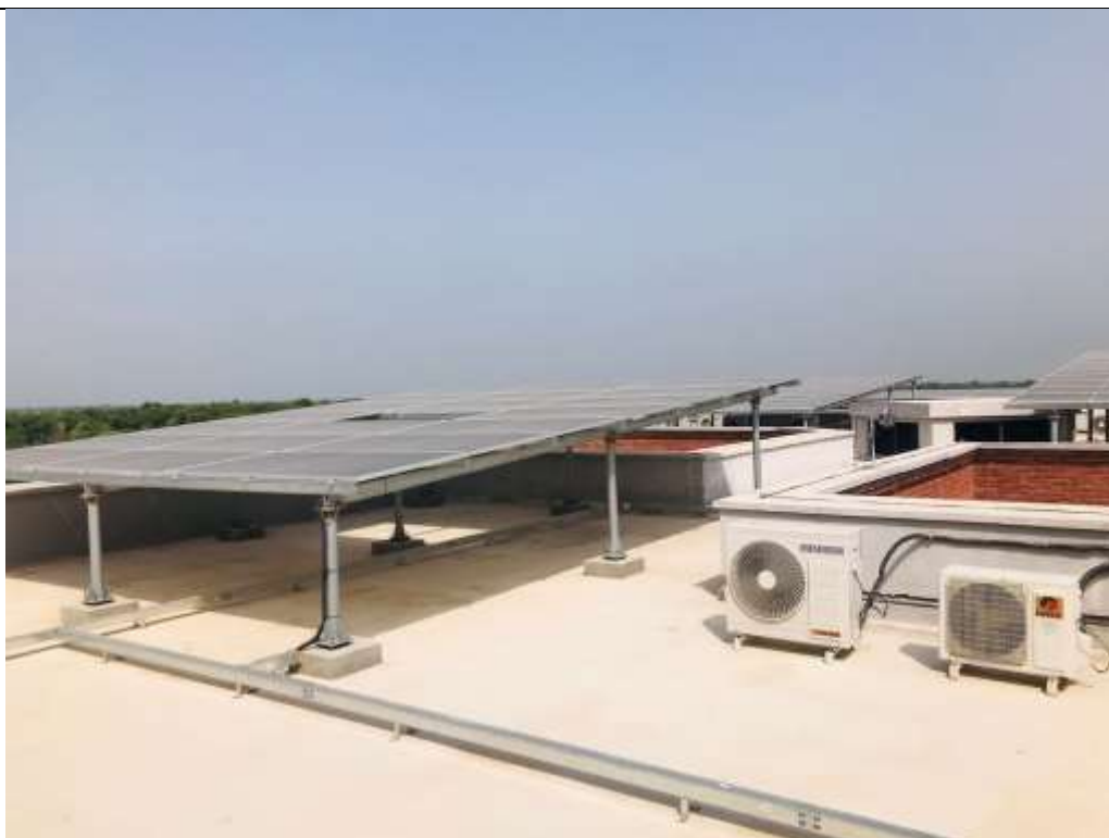
Solar Plates installed at Acadmic Block, Boys Hostel and Bus Shed roof top producing 45000 of units per month
